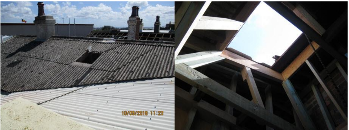
Images of where the asbestos roof sheeting gave way from outside and inside the residence.
