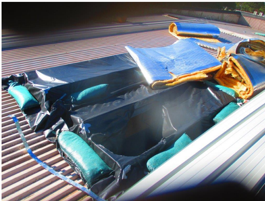
Image of the roof penetration the injured worker fell through.
