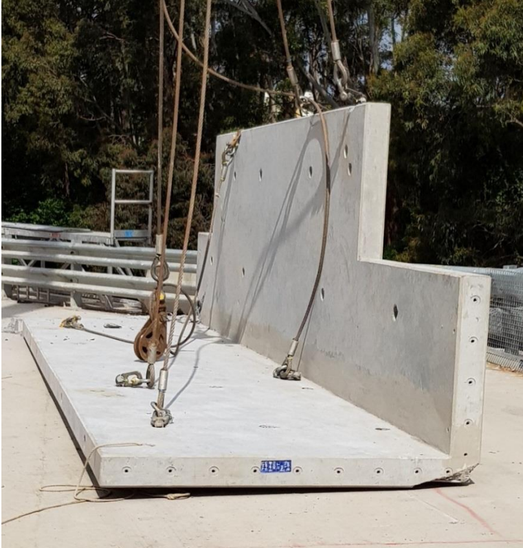
Image: A prefabricated concrete panel that dropped during installation.
