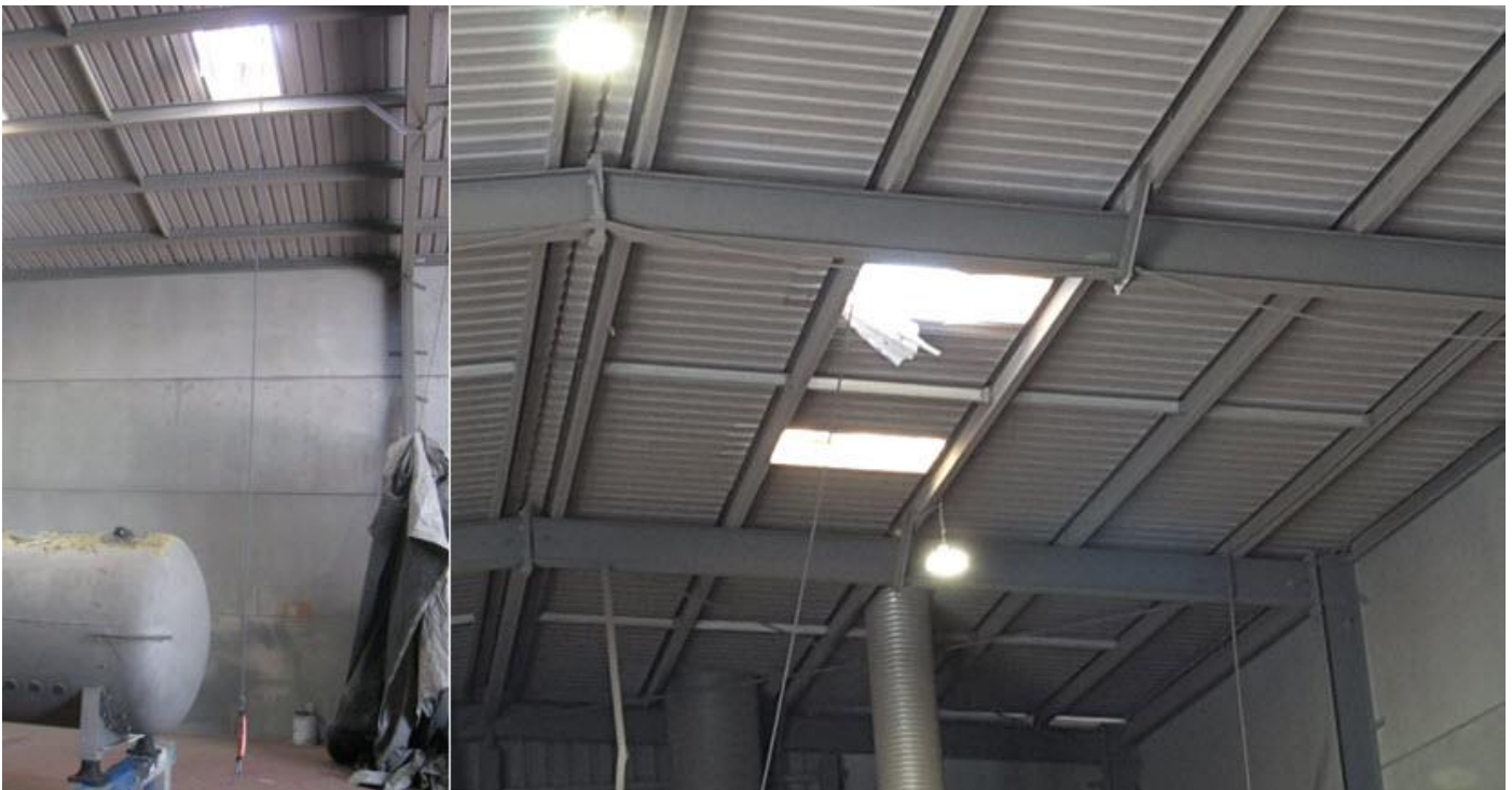
View of the broken roof sheeting from within the building.
