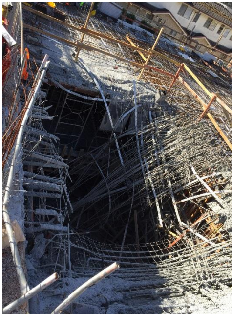
Image: Construction site showing where the collapse occurred.
