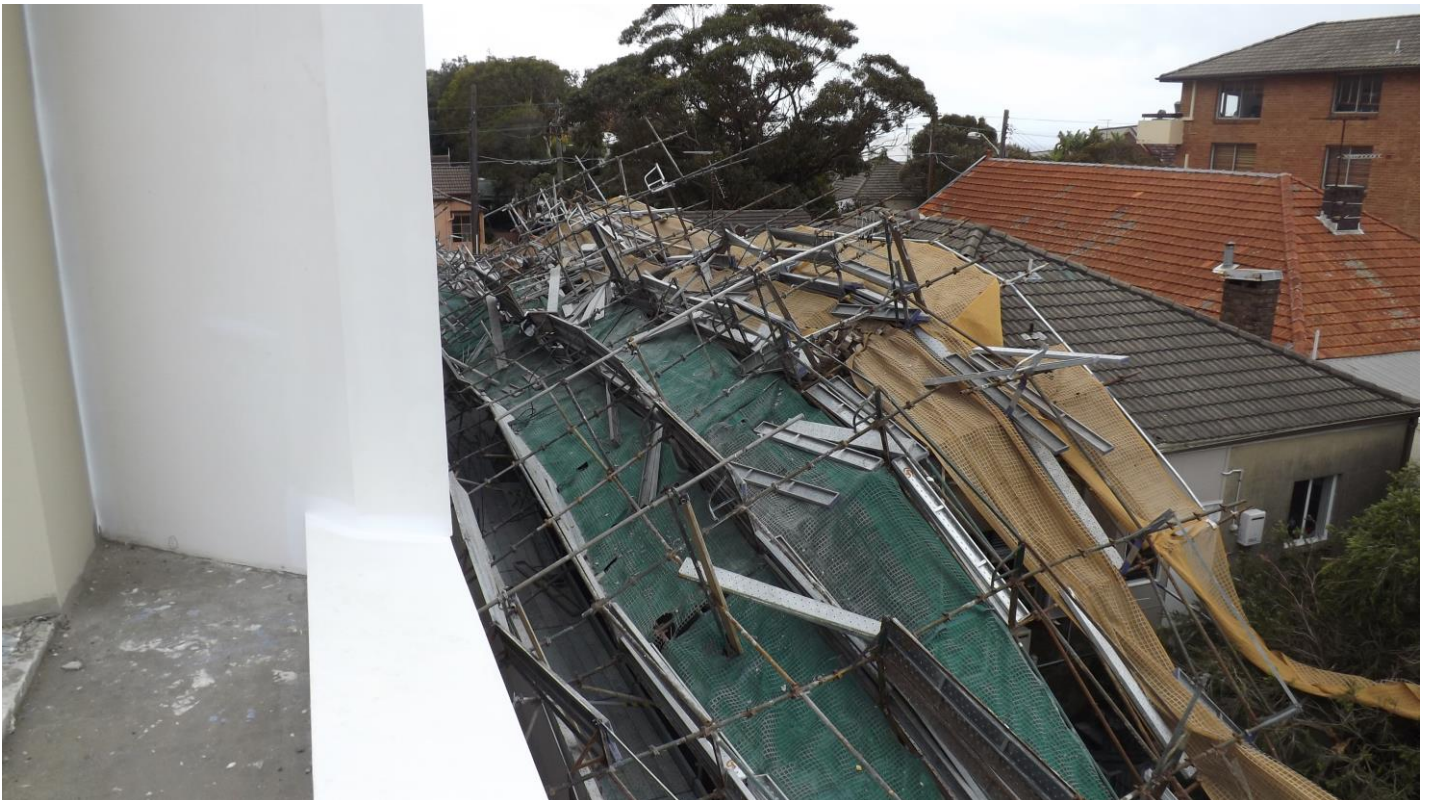
View of the 4-storey scaffolding which has collapsed and fallen onto a neighbouring property
