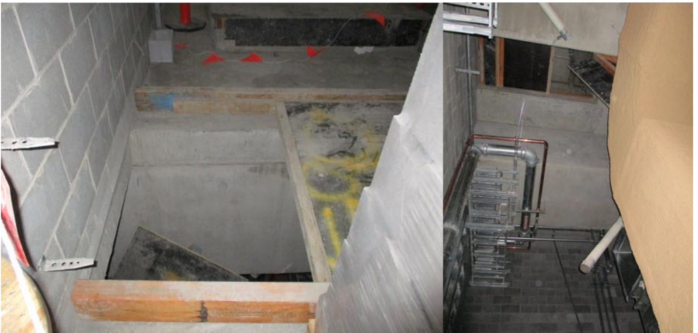
Image 1 & 2. View of open penetration from the plant room where the worker has fallen through and view from the level below looking up at the opening.
