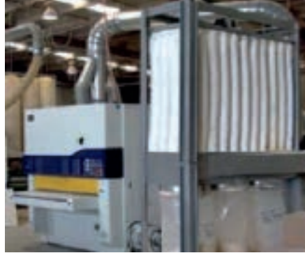
Local exhaust ventilation
